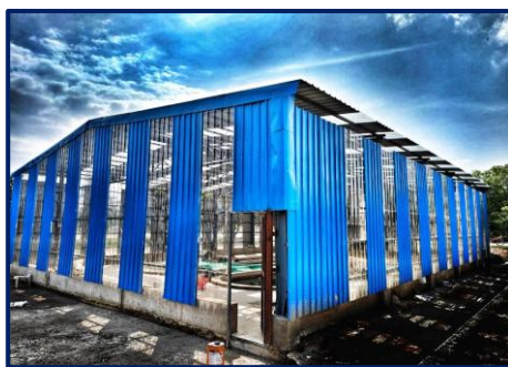
2 nos. Raceway Reactor at GAIL, Pata
