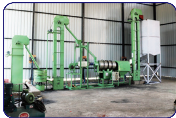
Mechanical Reclamation Plant
